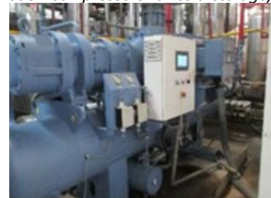
Screw refrigeration compressor for (IQF) conveyor, re-freezing
