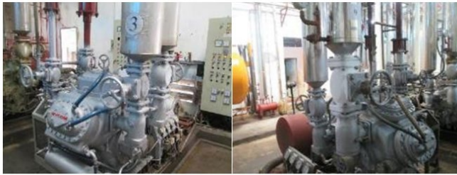
Existing reciprocating compressors
