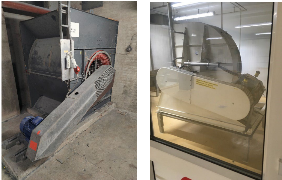
Figure 8 Example of belt-driven ventilators.
