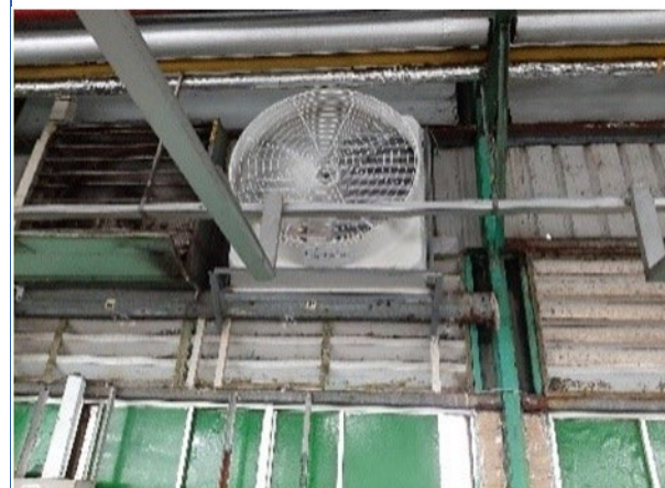
New fan (direct drive)
