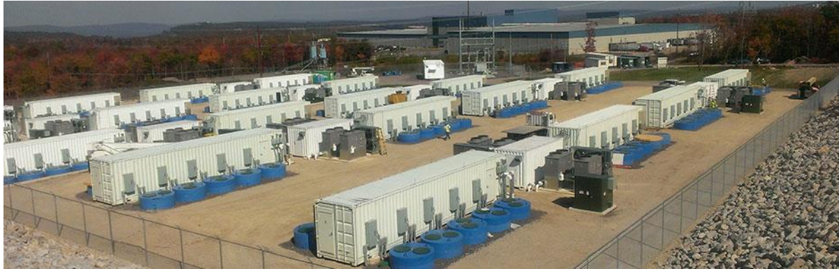
Figure 32: Photo of Beacon Power flywheel installation in commercial operation in PJM, Hazle, Pennsylvania. The plant includes 200 flywheel modules lowered into the ground (5 on each side of a container). The plant currently provides 20 MW of frequency regulation service to PJM and reached full commercial operation in July 2014 [6].
