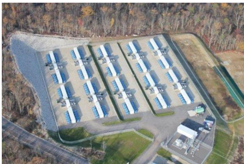
Figure 35. Beacon Power Hazle Township, PA plant 20 MW - 2013
