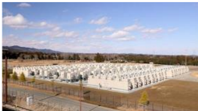
Figure 10: Picture of the 40 MW and 40 MWh energy storage system in Fukushima, Japan (Ref. 48).
