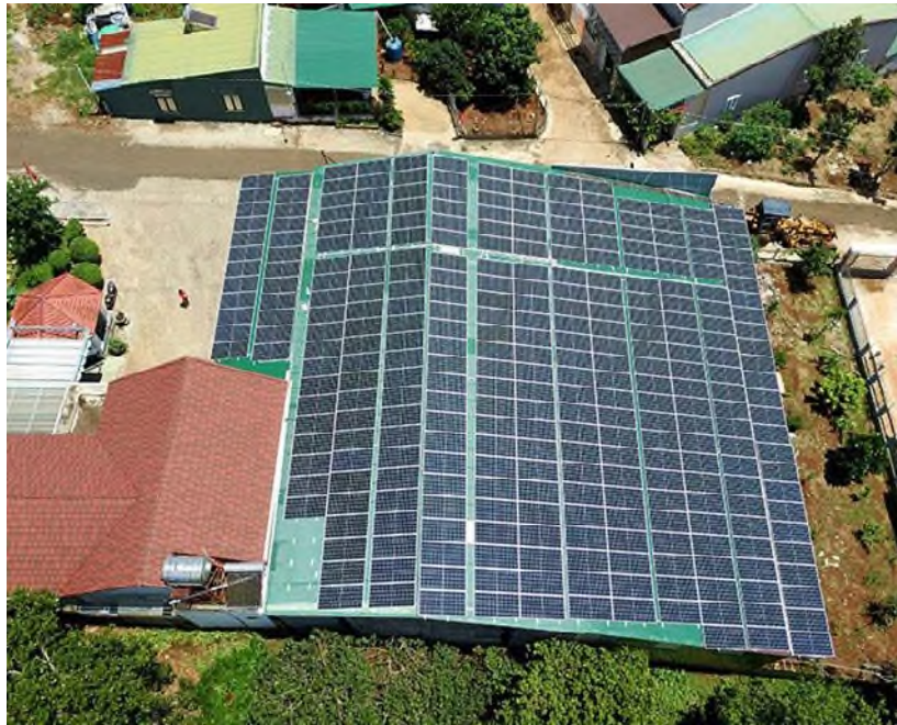
Figure 45: PV solar rooftop in Dak Nong province (135 kWp)
