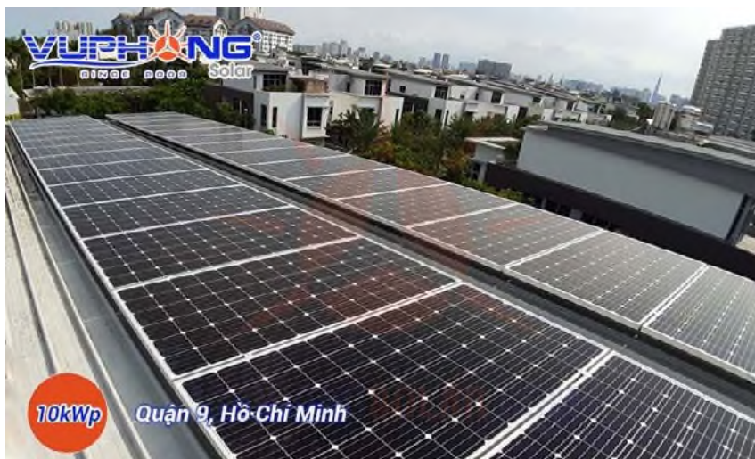
Figure 44: PV solar rooftop in District 9, Ho Chi Minh city (10.08 kW p )
